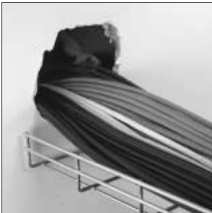
1. Existing hole with cables. Irregular hole cut.
