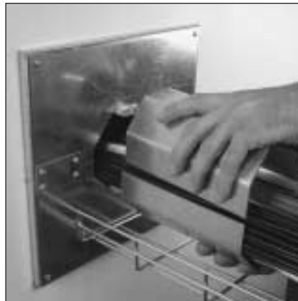
2. Attach ceramic heat protected wall plate to cover irregular hole cut. Insert split conduit around existing cables.
